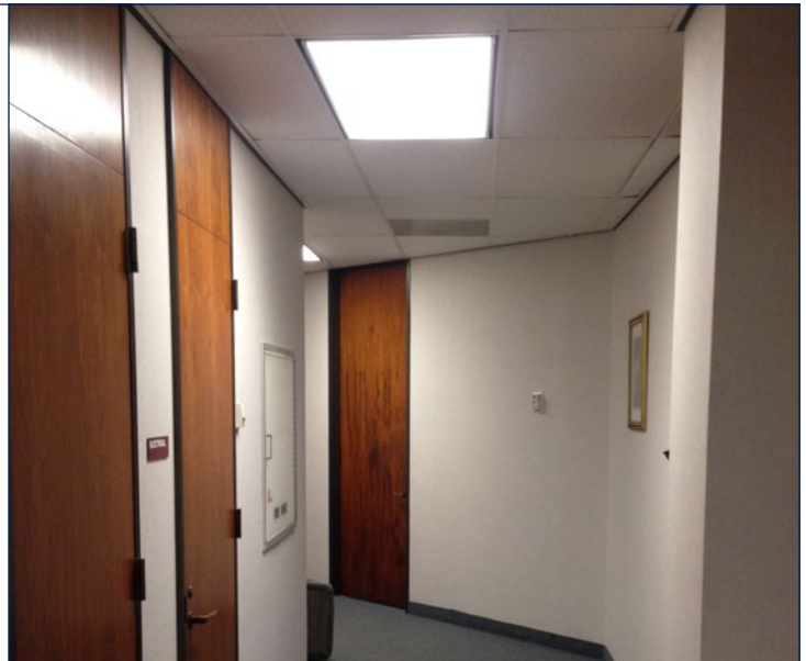
Figure 2: A lighting retrofit included installation of T5 fixtures with reflectors and an overall reduction in the number of fixtures in tenant common spaces.
