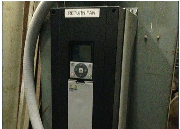
Figure 4: A new return fan and controls were among a package of HVAC retrofits installed in early 2012.
