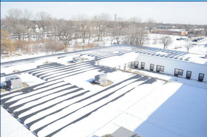
Figure 2: The largest of the three solar photovoltaic systems installed on the apartment rooftop.
