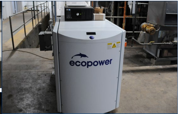
Figure 5: A 4.4kW DC-rated ecopower micro-combined heat and power system.
